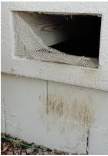
Broken screen in housing foundation
