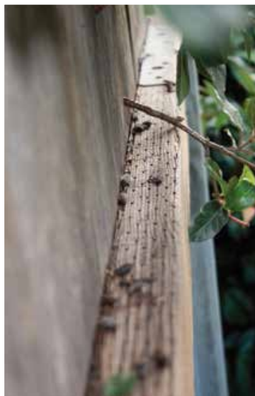
Known rodent runway: Evidence of droppings along fencing.
