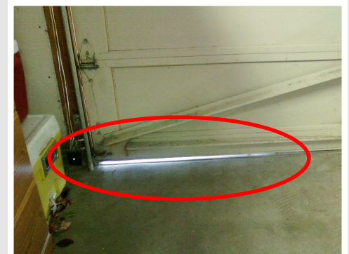
Gaps under doors can allow rodents to enter structures.
