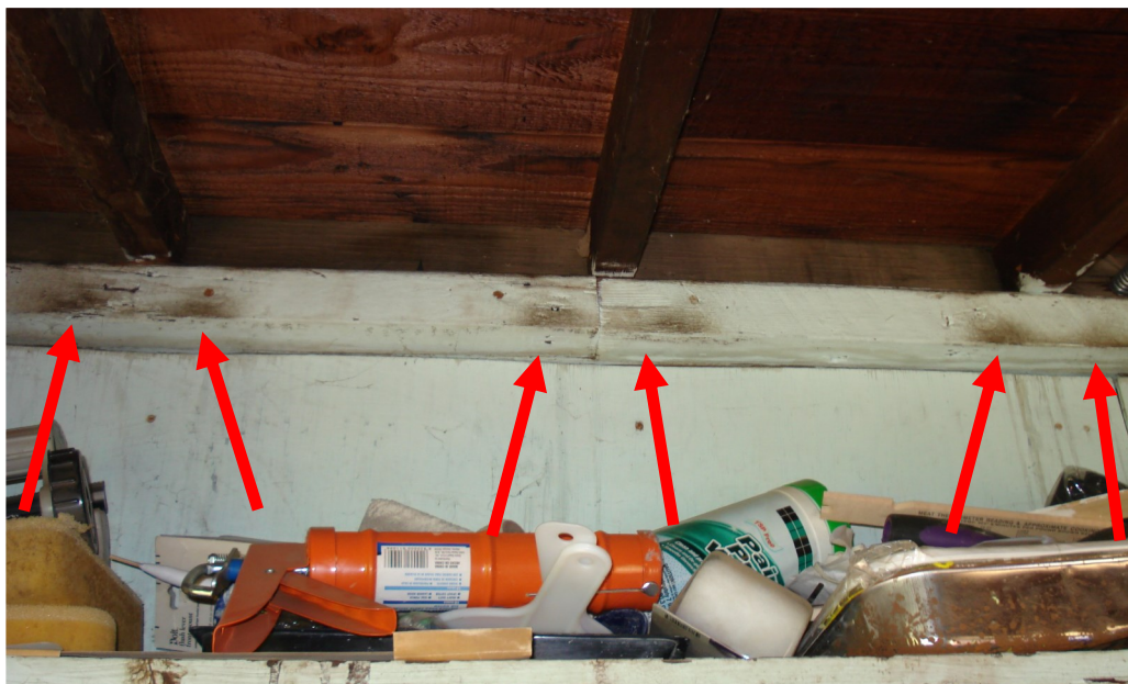
Rodent Activity: Grease rub marks around the roof beams in an outdoor shed.
