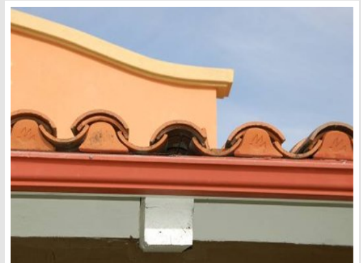
Missing end caps allow for rodent harborage.
